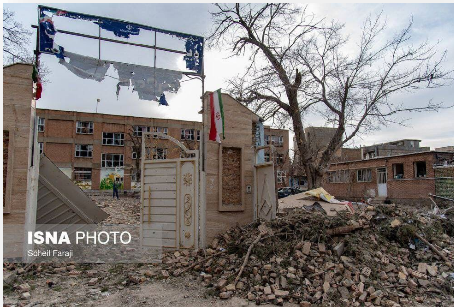
The Imam Reza boys' school in Abyek, Qazvin, was seriously damaged. An innocent schoolboy was killed and 3 of his schoolmates were injured.
